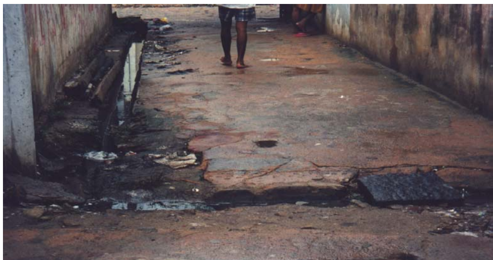
Plate 4.6. Broken section of drainage channel
