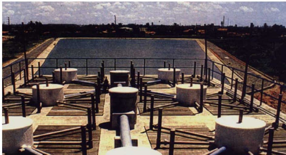
Plate 4.49. Mangueira Sewage Treatment Plant
