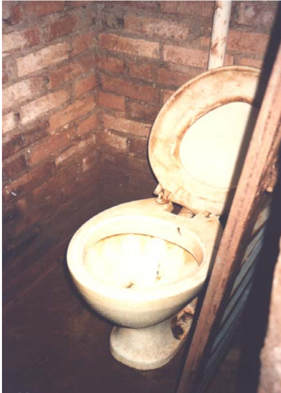
Plate 4.22. Low-volume flush toilet
