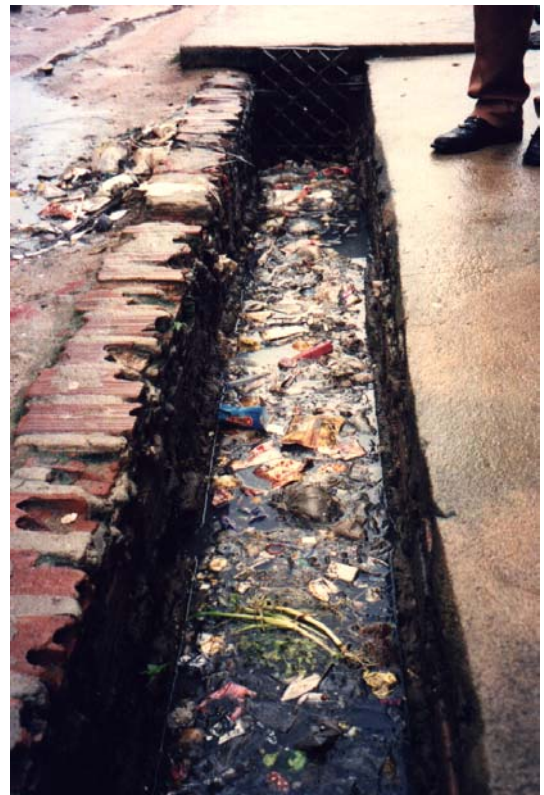
Plates 4.10. Presence of solid waste in the drainage channels
