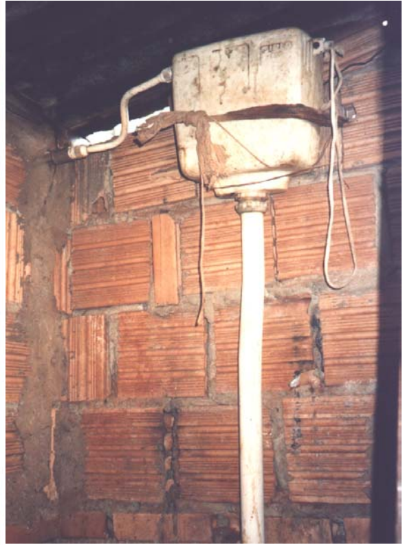
Plate 4.23. High level cistern
