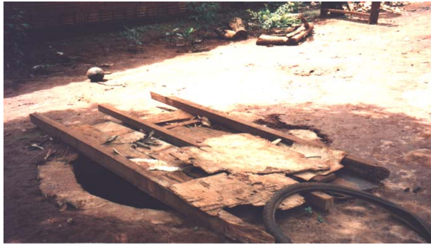
Plate 4.28. An improvised pit cover
