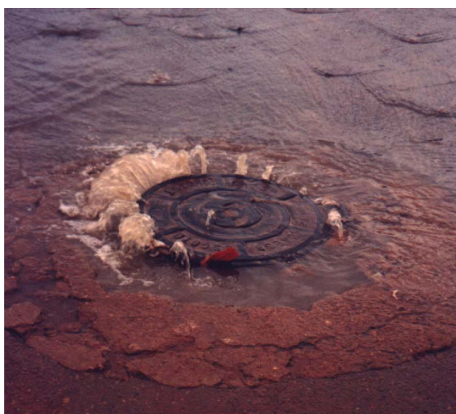
Plate 4.48. Manhole overflowing after a rainy night
