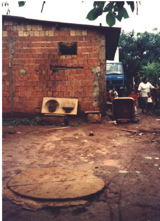
Plate 4.26. An in-house bathroom connected to the leach pit
