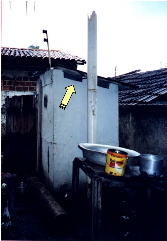
Plate 4.15. The original ventilation designed for the latrines
