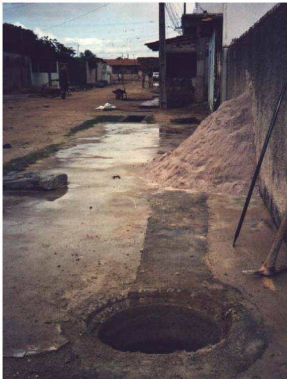
Plate 4.59. Three clogged inspection chambers
