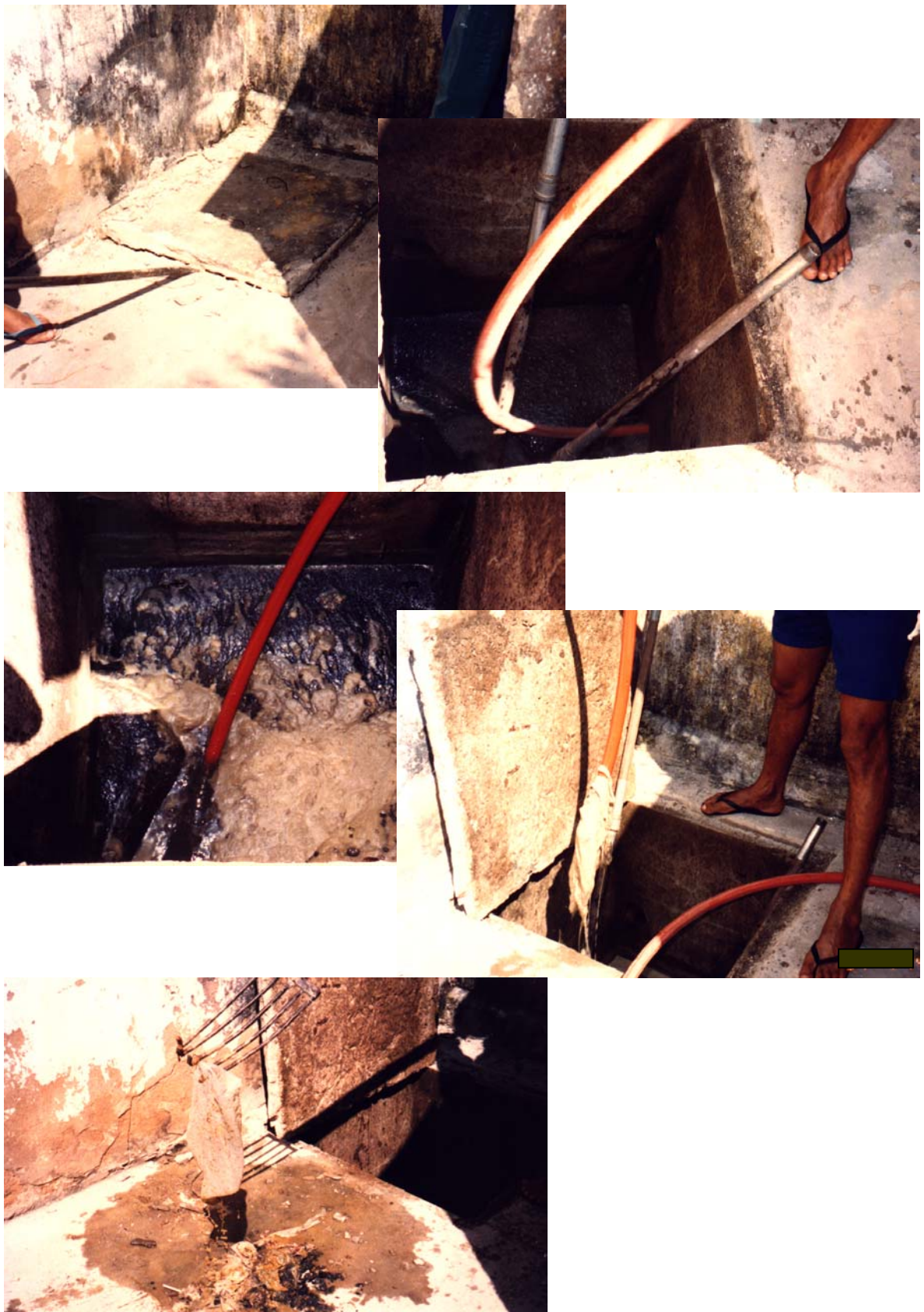
Plate 4.34. Sequence of photos showing cleaning out of a condominium sewer which had been blocked by a piece of cloth and a plastic bag.
