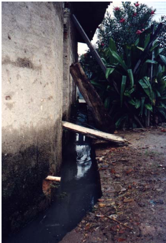
Plate 4.9. Clogged drainage channel
