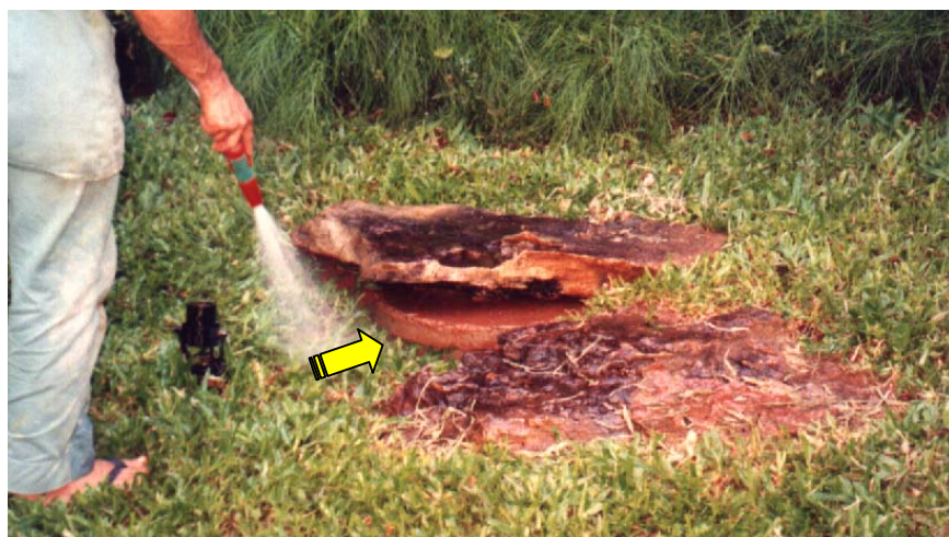
Plate 4.39. The inspection chamber of a backyard layout condominial sewer integrated to the garden design of a property in the high-income area of Lago Norte.
